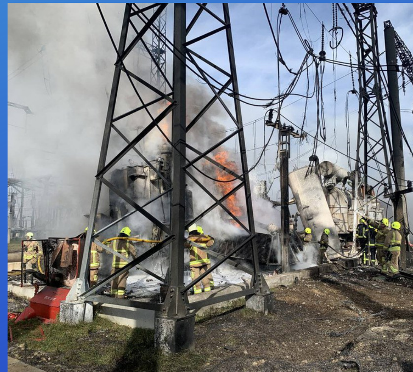
POWER ELECTRICAL SUBSTATIONS
